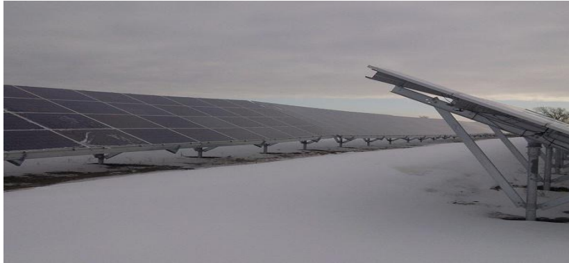
Figure 7. Typical row of solar panels in winter showing very little to no snow accumulation around foundation piles
