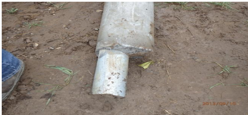
Figure 10. Pile moved into soft soil before concreting
