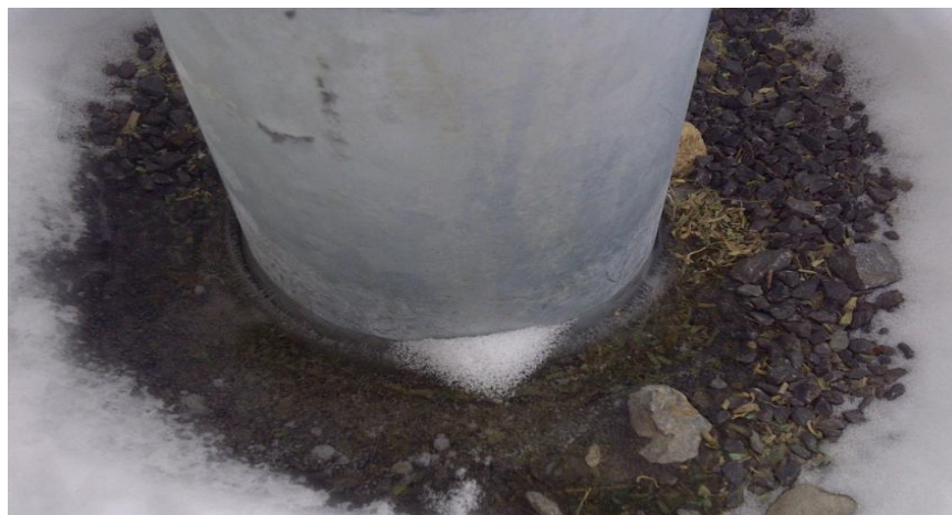
Figure 8. A pile moving out due to frost
