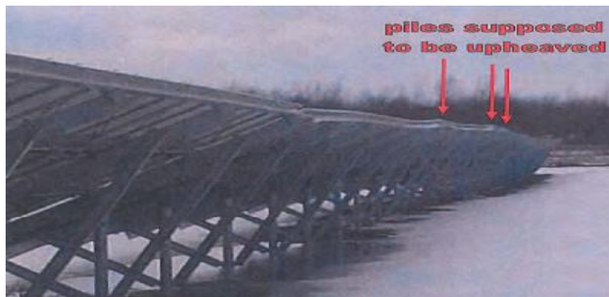
Figure 9. Piles affected by frost showing deformation of the racking
