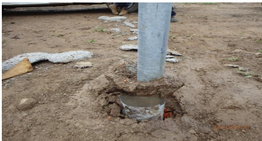
Figure 11. Pile failure in uplift in load testing in soft soils
