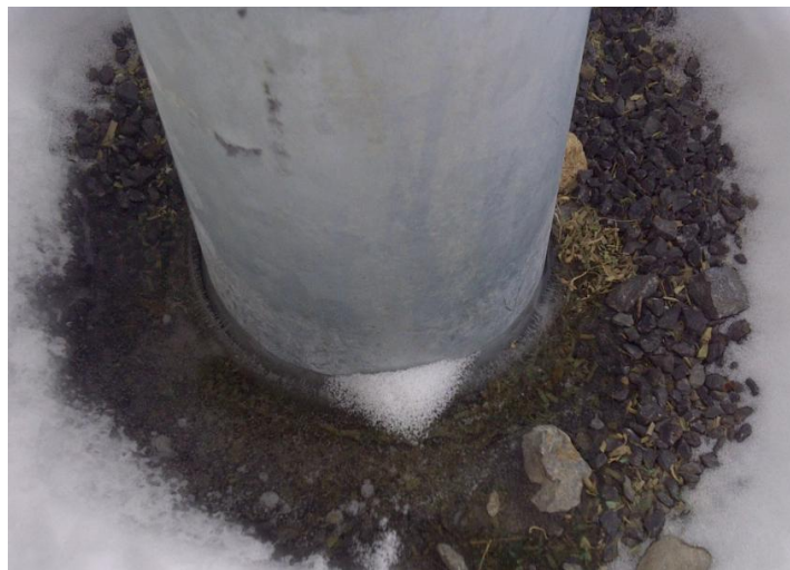
Figure 2. A pile moving out due to frost
