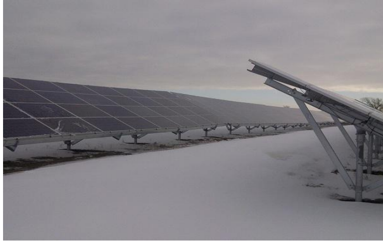
Figure 1. Typical row of solar panels in winter showing very little to no snow accumulation around foundation piles.
