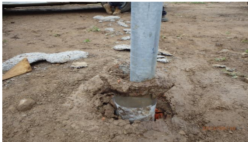
Figure 5. Pile failure in uplift in load testing in soft soils
