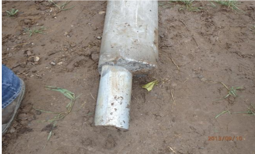
Figure 4. Pile moved into soft soil before concreting
