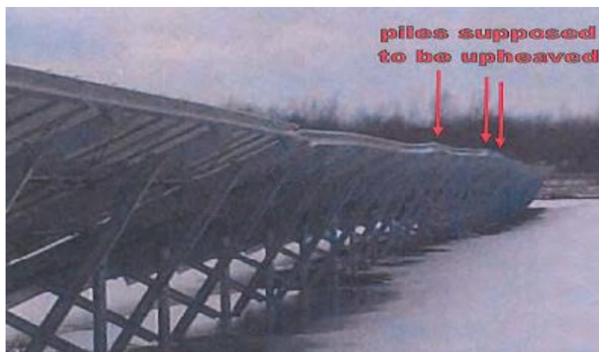
Figure 3. Piles affected by frost showing deformation of the racking
